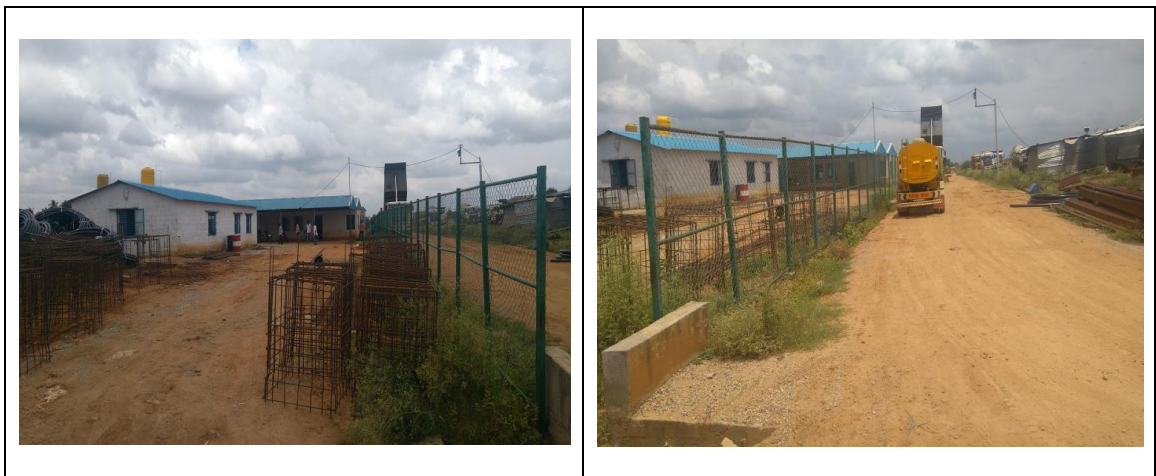
Exhibit 3.1: Chain link fencing work executed at Sy.no. 121, which was not part of the approved survey numbers
